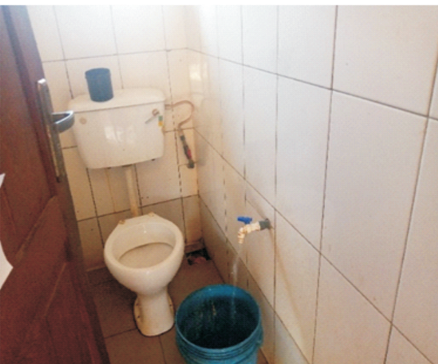
Plate 5: Flush toilet at Ogida toilet facility
