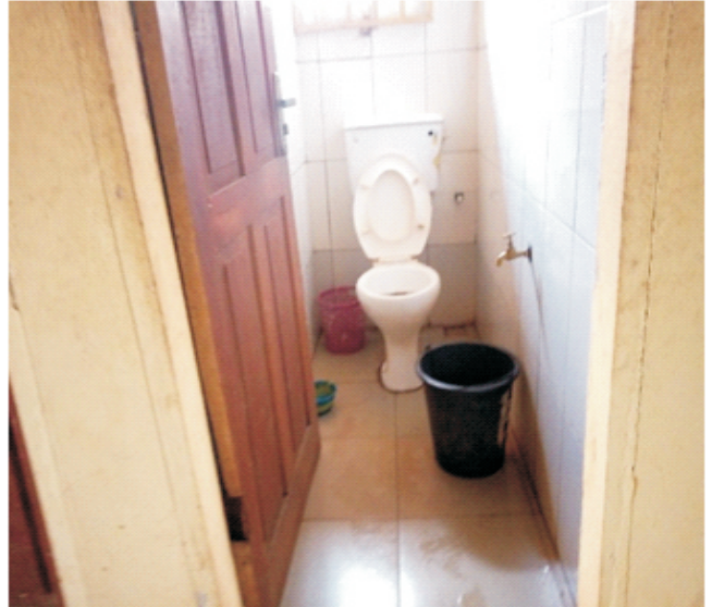
Plate 2: Flush toilet at Uselu market toilet facility
